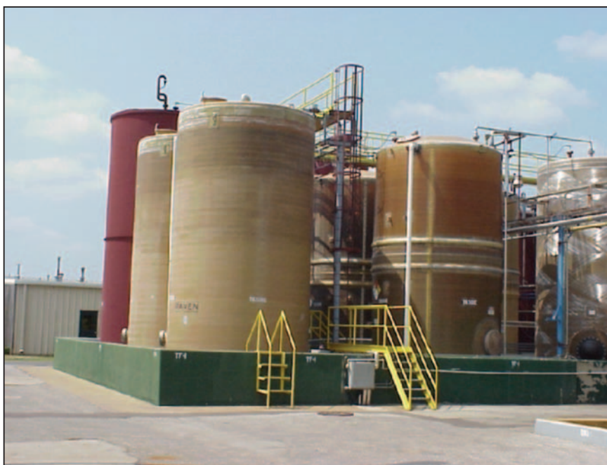
FIGURE 1. Tank farms at facilities should be treated as high-risk areas for potential accidental chemical releases
