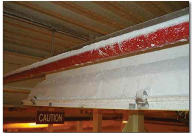
Photo 1: Dust accumulating on overhead surfaces.
