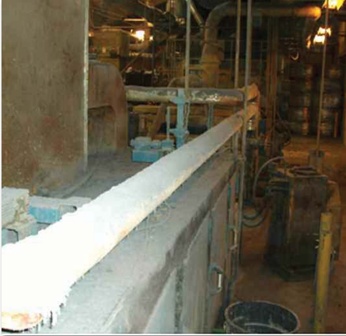
Photo 3: Phenolic resin dust accumulation due to inadequate dust collection.
