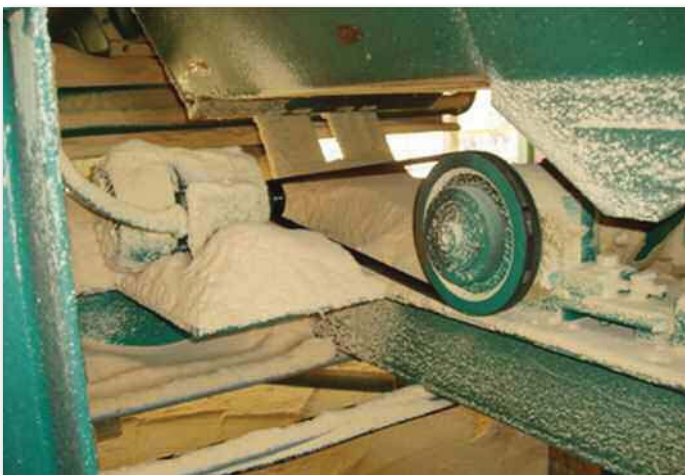
Photo 2: Dust leaks at a material transfer point in a wood planer mill.
